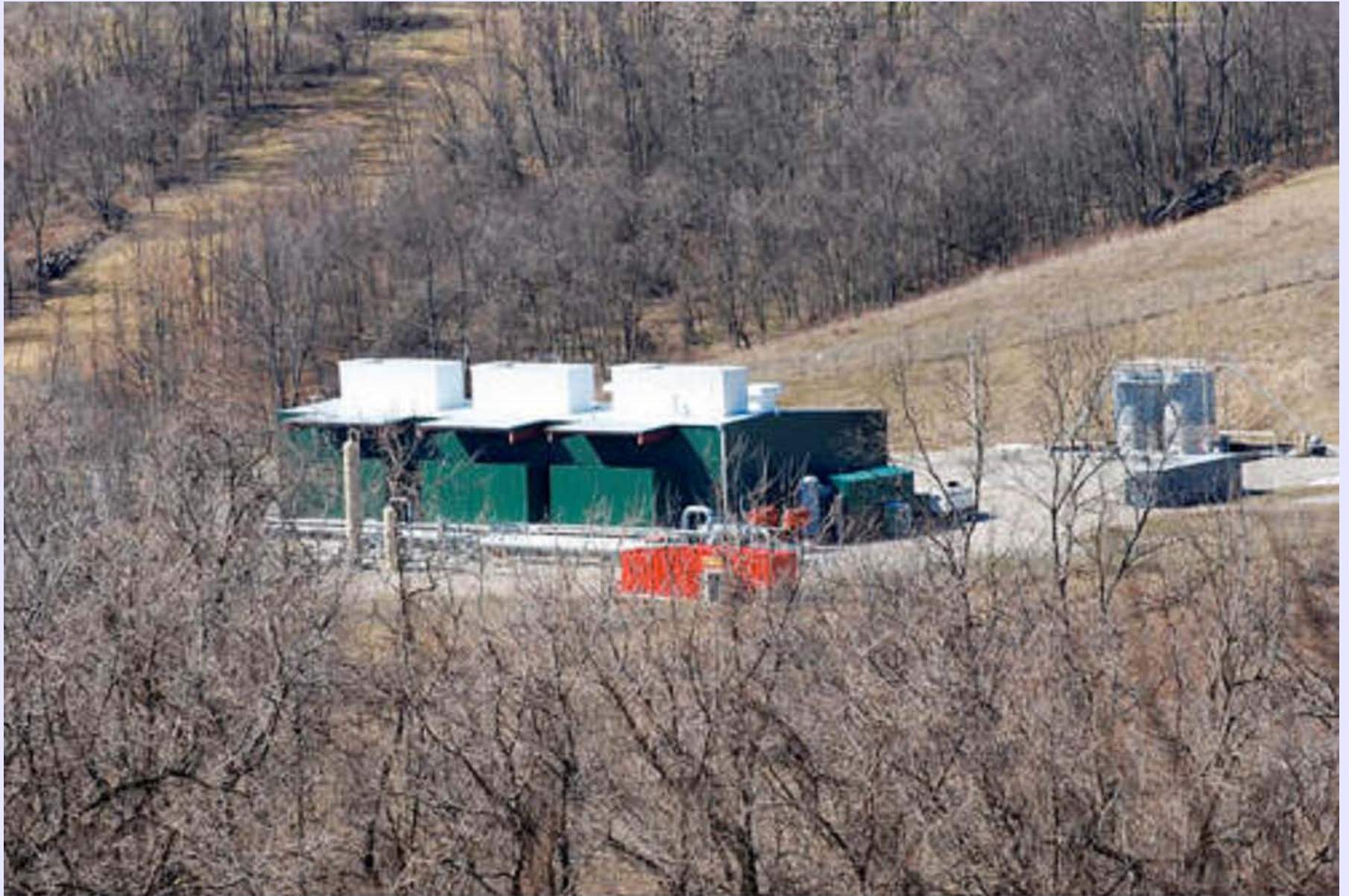
Dryer Compressor Station March 2011 Expanded to 3 compressors
